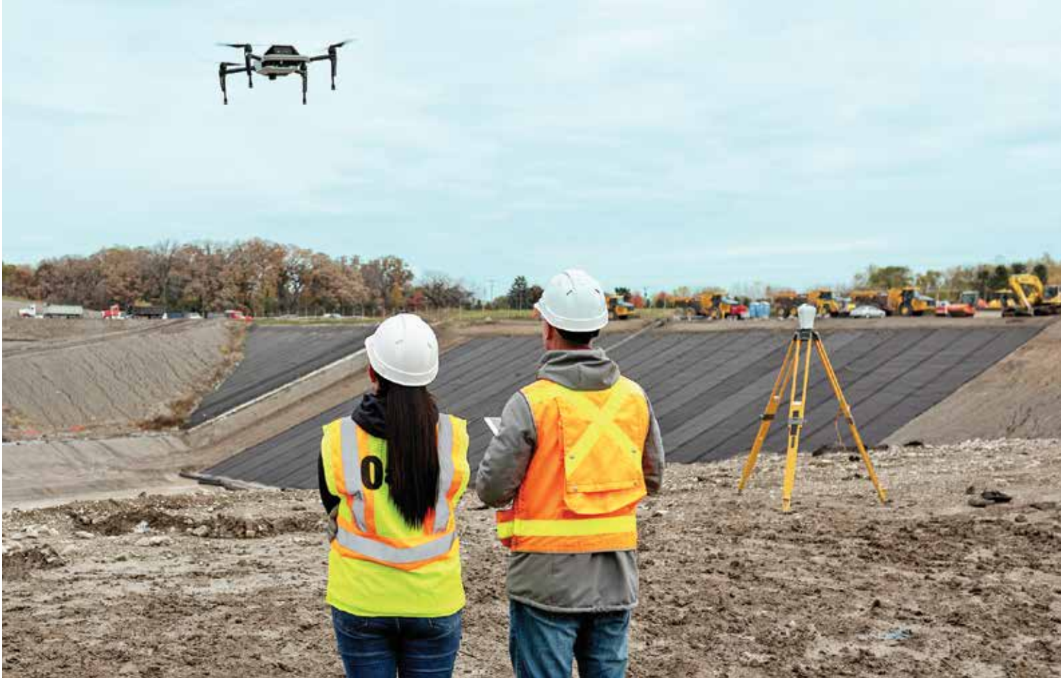
Automation between humans and machinery is increasing job site efficiency. Drones and GPS technology are among the technologies making it happen.
