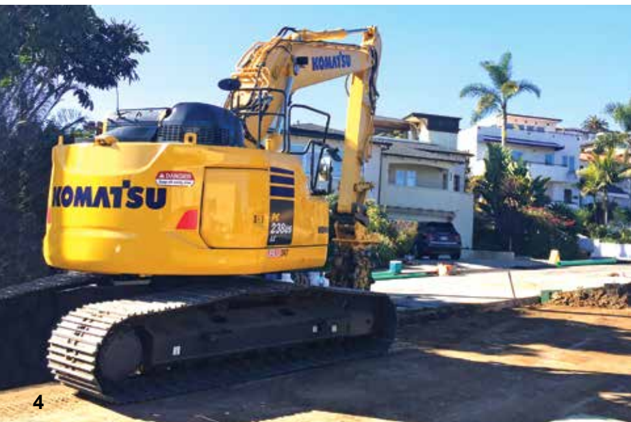
KTA Construction puts its new Komatsu PC238USLC excavator to work on the City of San Diego Sewer & Water Group's 764A project near Point Loma.
