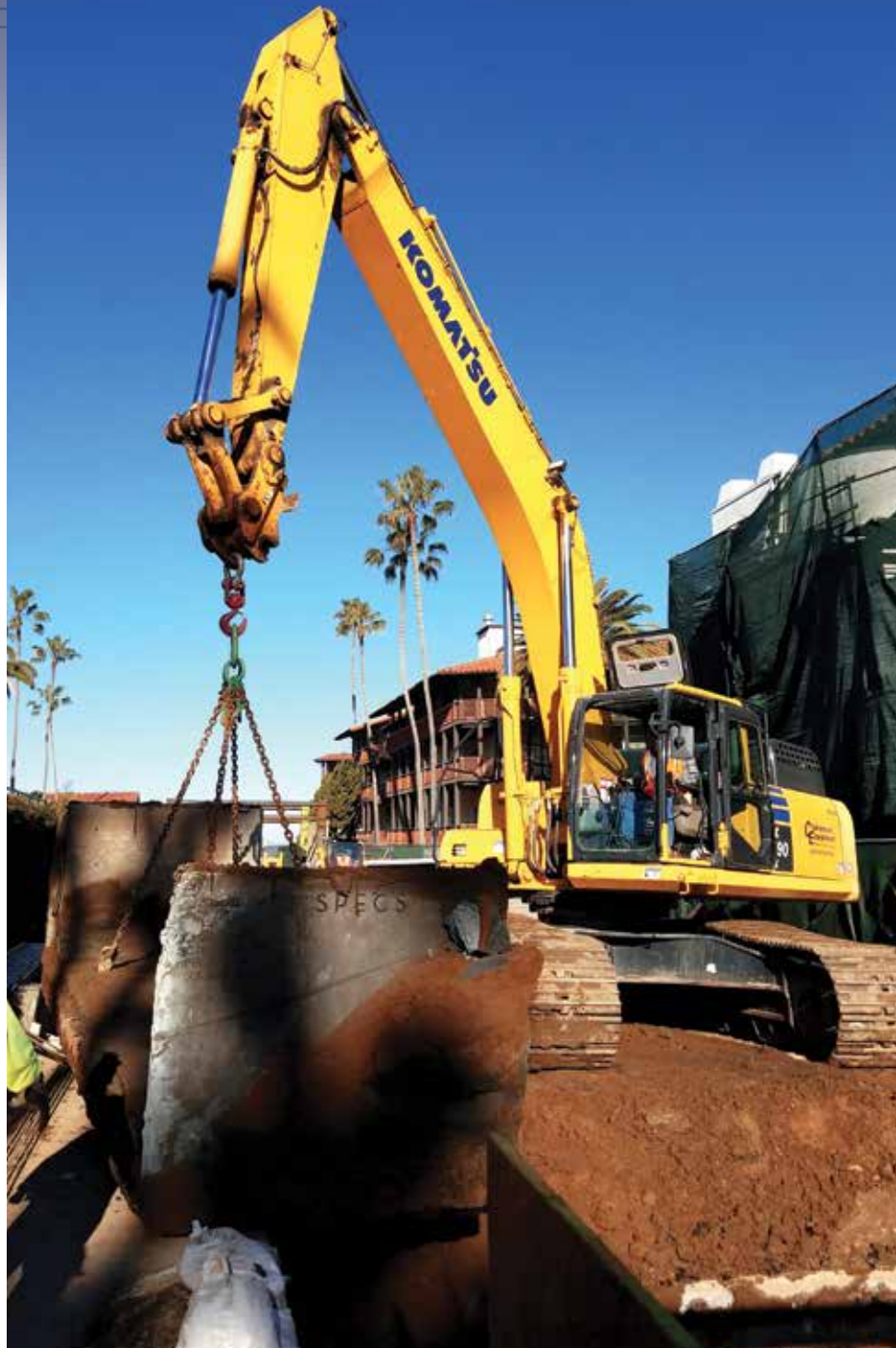
Operator Curt Hendrickson removes a section of a pre-cast box culvert on the La Jolla Avenida De La Playa storm-drain replacement project with a Komatsu PC490LC excavator.
