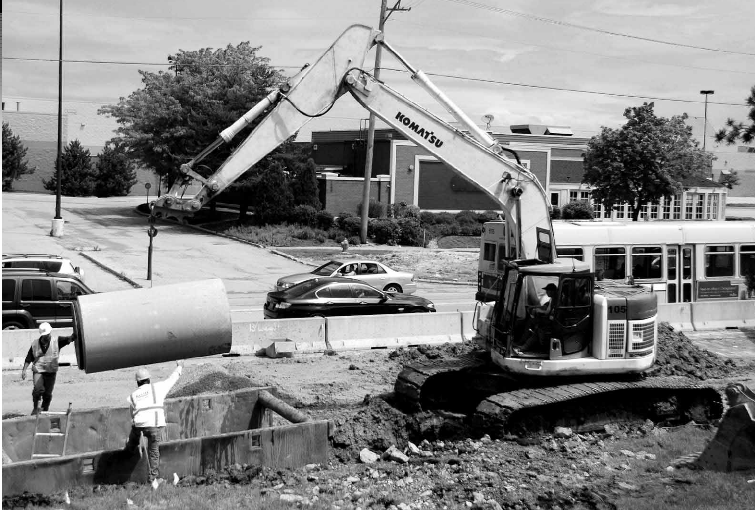
Figuring operating costs can be challenging because a particular machine may perform multiple tasks, such as an excavator that's used to dig and set pipe. Contractors must consider how each application affects production and fuel usage, and use other critical information to better calculate accurate operating costs.
