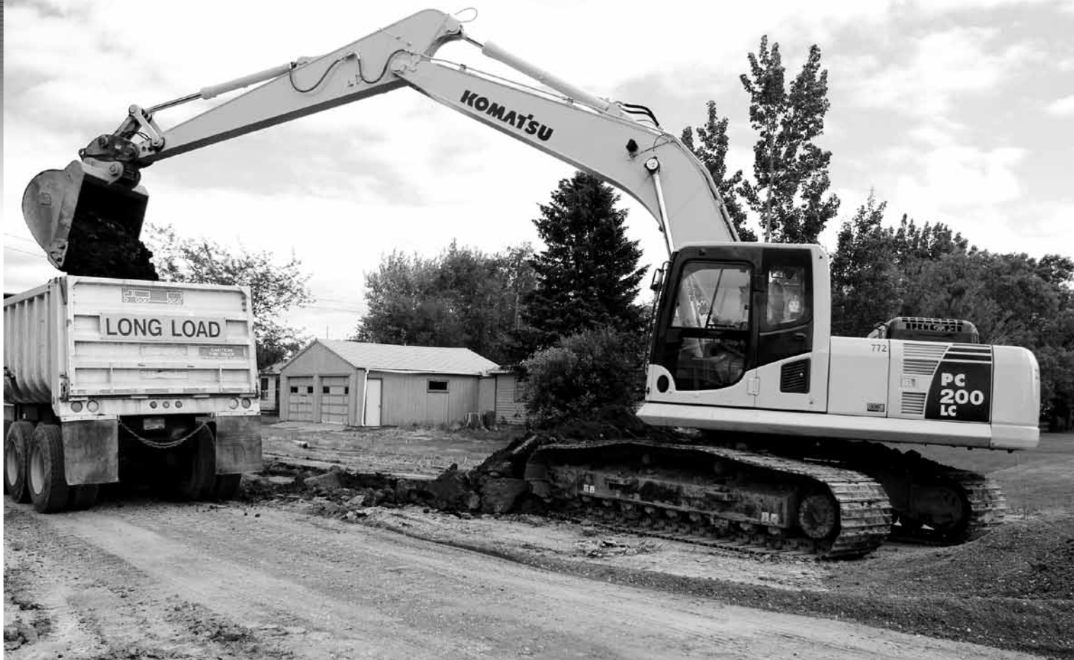
There's a push to use less virgin material and more recycled material in new-road construction. The Greenroads Foundation developed a rating system for Greenroads certification, much like LEED certification for buildings.
