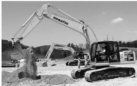
Attendees could operate all types of Komatsu equipment, including the new Hybrid PC200LC-8 excavator and the PC270LC-8.
